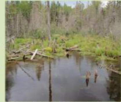
Water ponded upstream of an old crossing is a good indication that the crossing is set too high.
