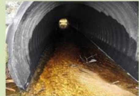
A culvert installed to stream smart principles that is accumulating substrate
